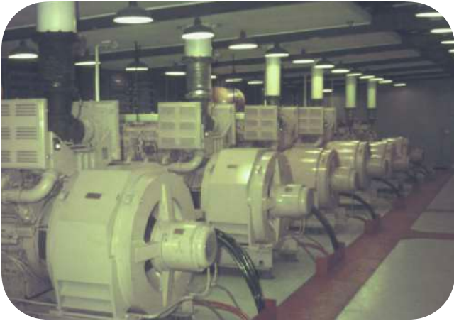
The generators in the onsite power station that consumed the fuel to power the Tracking Station and associated communication network
