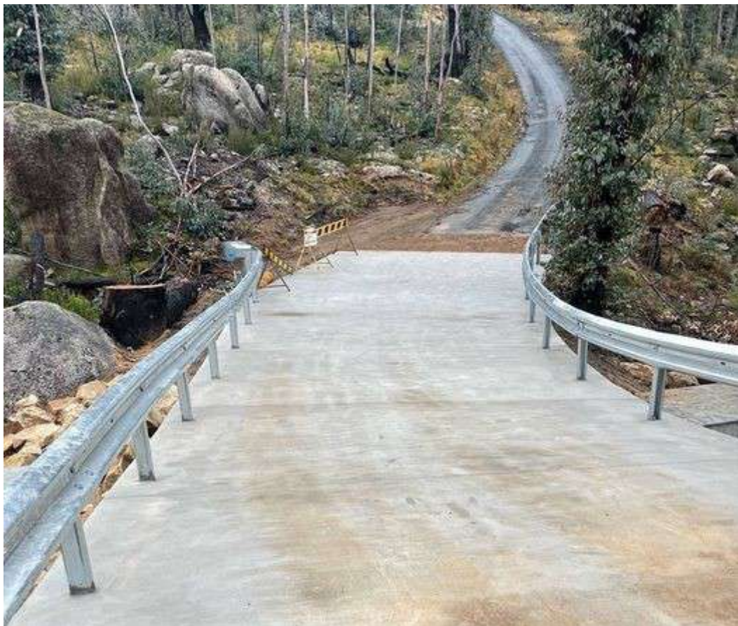
The new culvert/bridge on the reopened road to Booroomba Rocks car park
